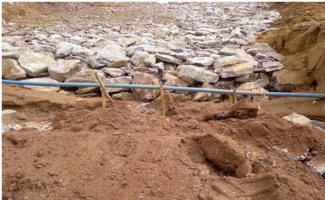
Rock fill No:1 @ Bambisa Drive and Preparing for the protection of the existing water main pipe.
