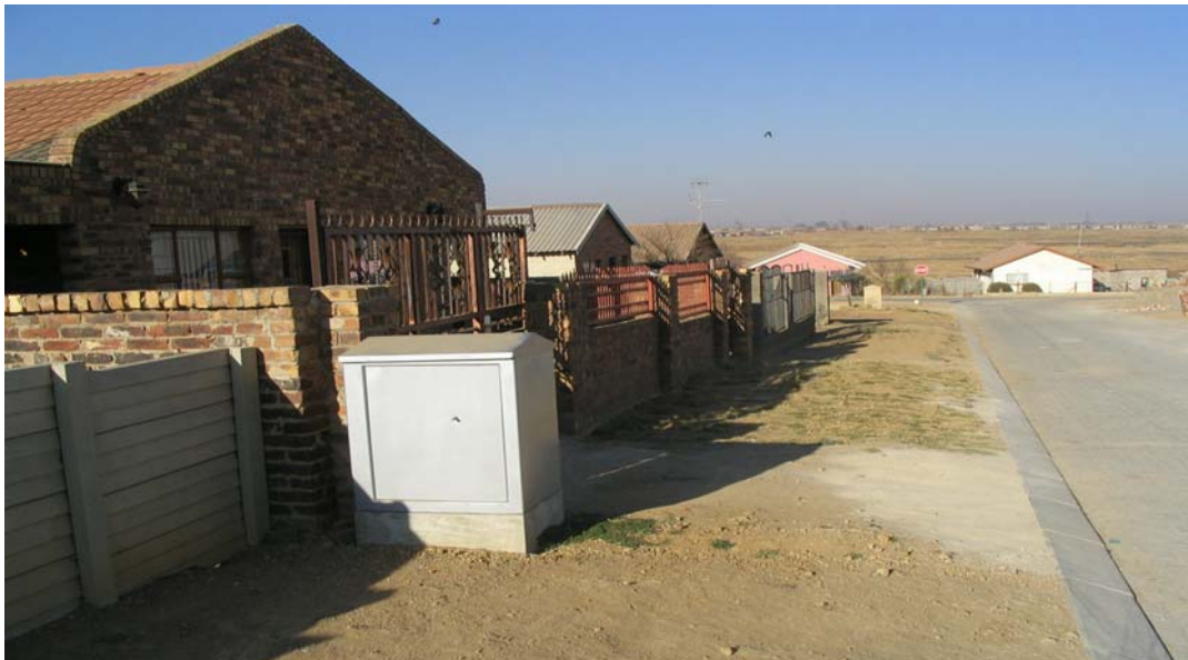
Meter kiosks are protected to prevent consumers from stealing electricity
